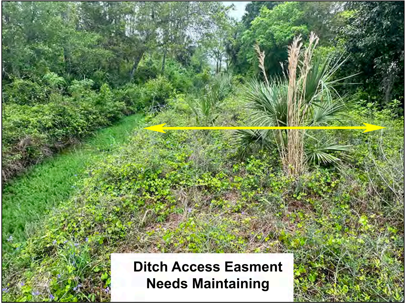
Figure No. 4 - Ditch easement area needing maintenance to provide access to the ditch system.
